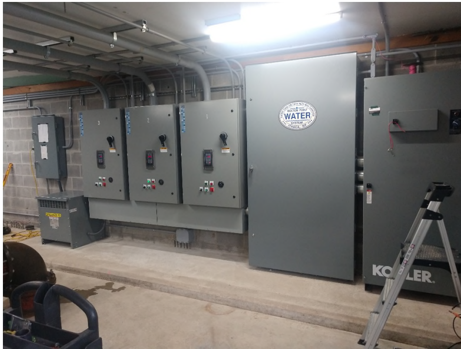
New pump soft starters, main panel, and transfer switch at Oakcrest Booster Pump Station
